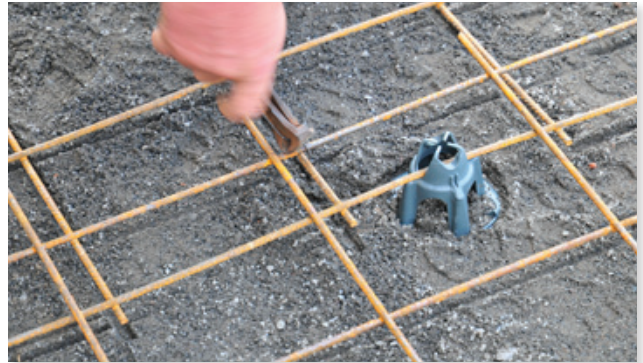
The double wire along the edge of the steel is a lot stronger to tie together and reduces wastage because you don't over exceed lapping, so you get more steel for your money.
